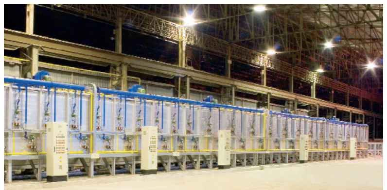
Fig. 3 Vesta tunnel kiln
